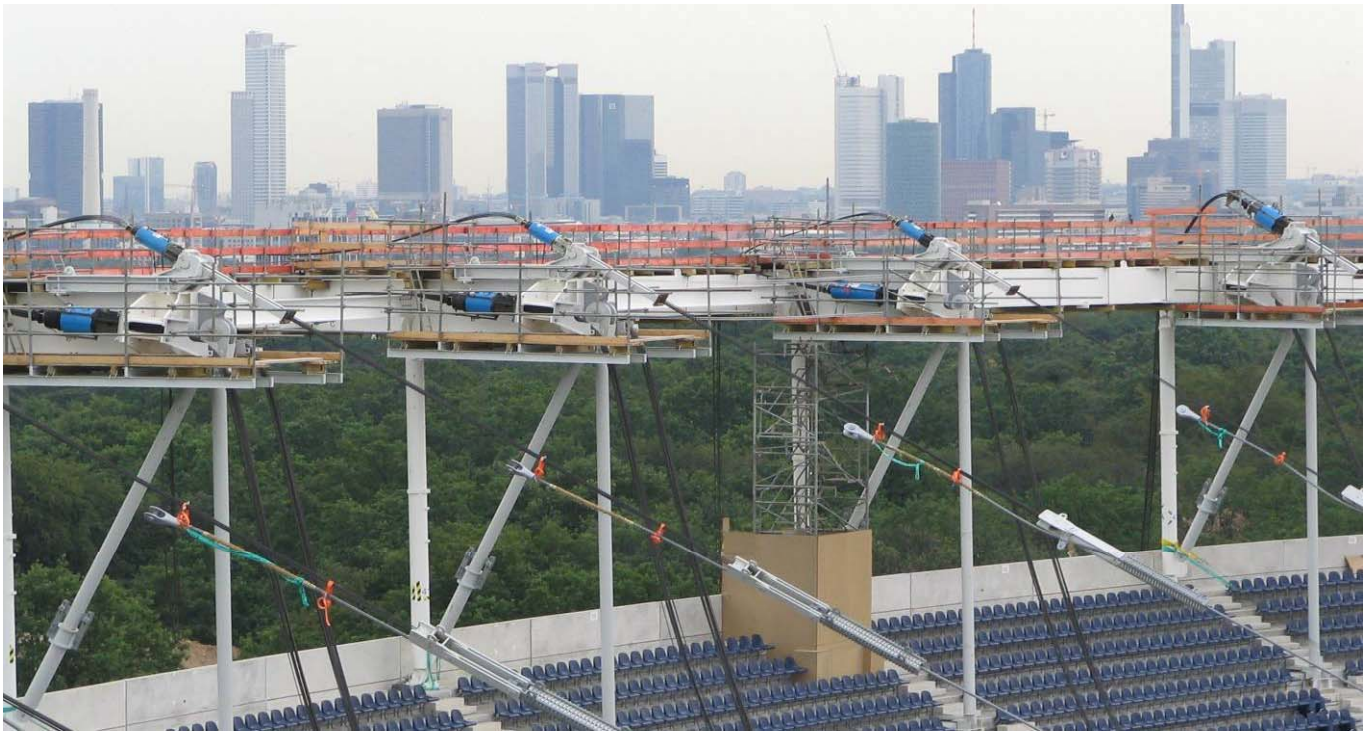
▲ Partial view during the first pulling stage with the centre of Frankfurt in the background
